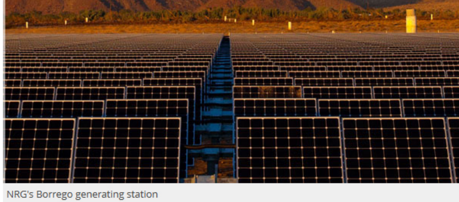
NRG's Borrego generating station
